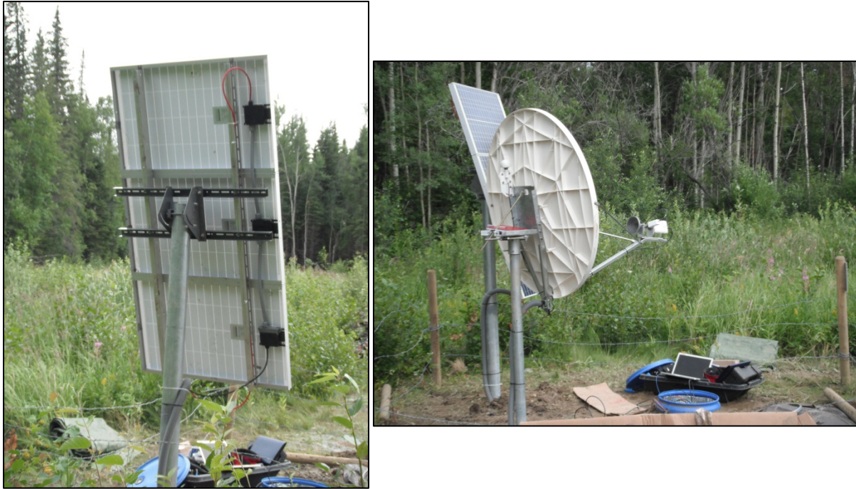
Figure 7. Pictures of mounted solar array (left) and satellite dish (right).
