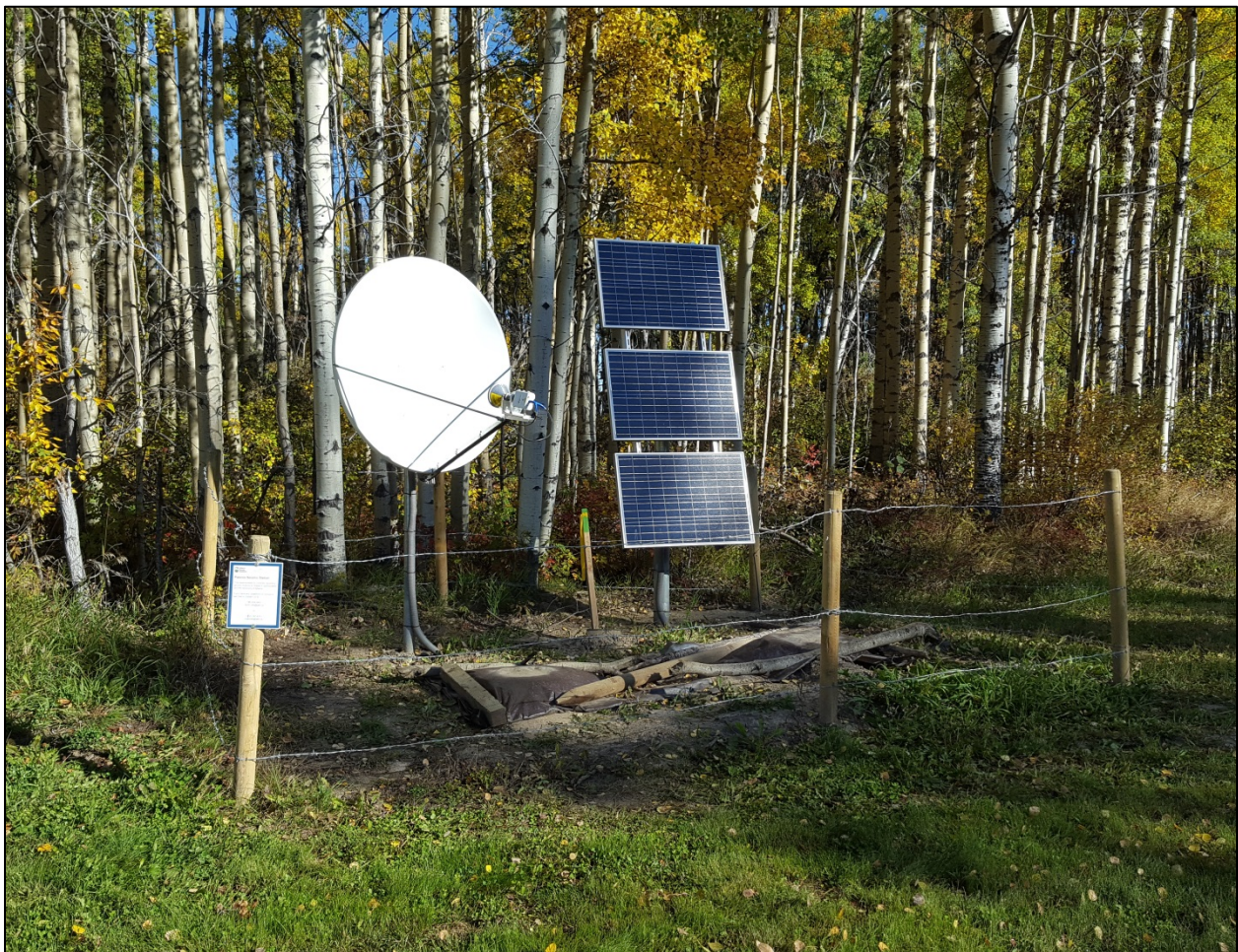
Figure 1. Completed installation of a RAVEN station.
