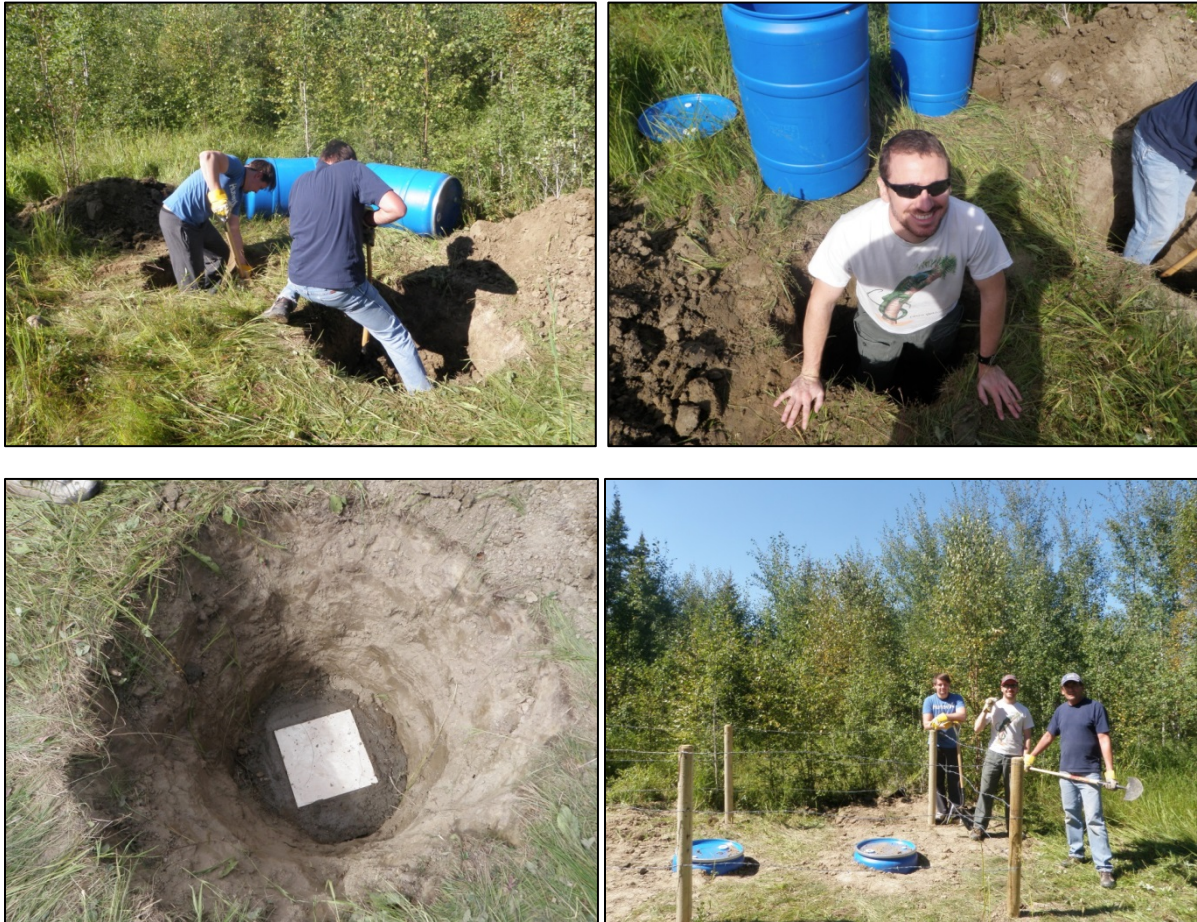
Figure 4. Installation of infrastructure. Left to right, top to bottom: digging vault holes, burial of vaults, cementing the seismometer pier, and fenced off enclosure. Not shown: solar and satellite mounts.
