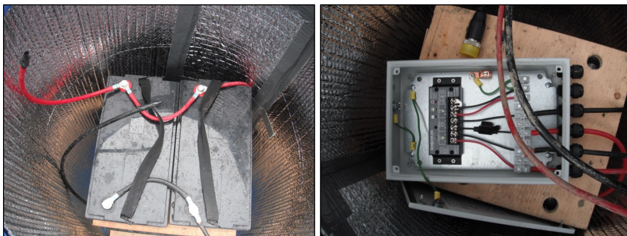
Figure 6. Pictures of battery bank wiring. Left: four batteries in place, wired in parallel. Right: regulator wired for the battery bank and solar panel. Ground cable and Cygnus power cable are not shown.
